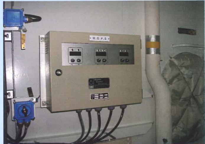
COPRON ELECTRIC PANEL
