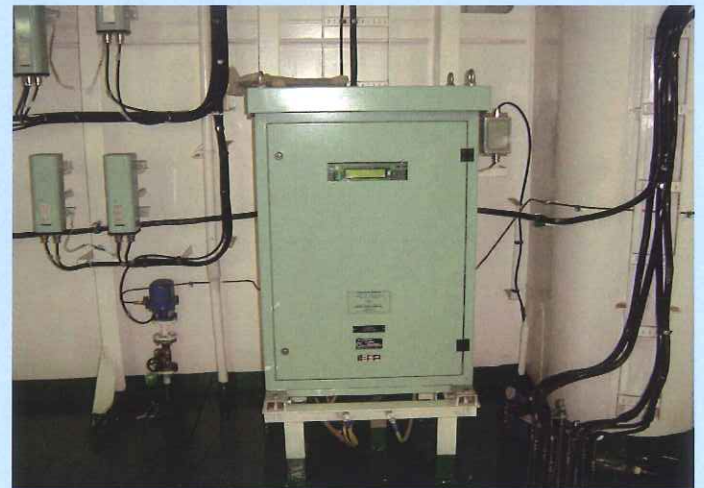
ICCP ELECTRIC PANEL
